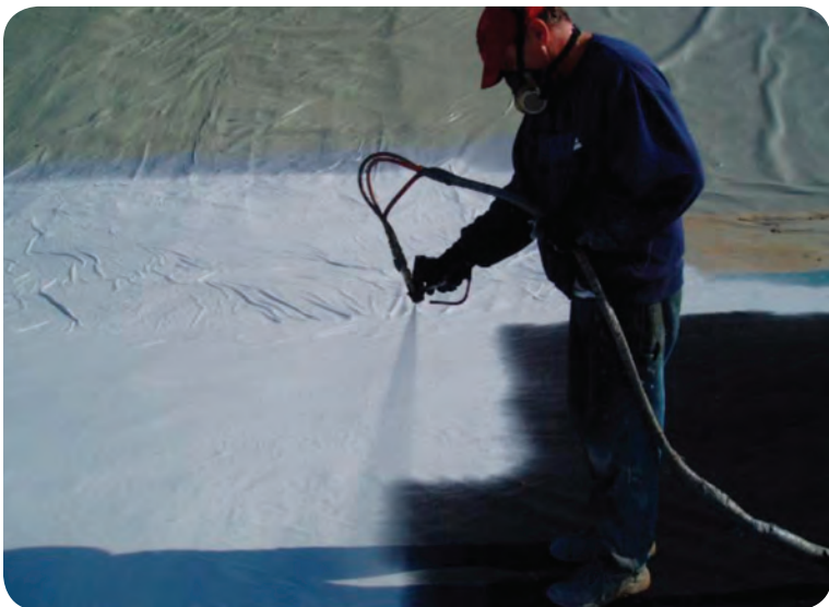
For containment areas where solid substrates are not present, geomembranes can be used with an applied layer of a polyurea system. Photo courtesy of GlasCraft, Inc.
