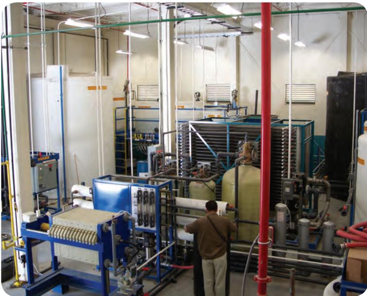
A water recycling system installed at a new finishing plant in Reynosa, Mexico, is minimizing water costs and providing a consistent source of high-quality water to the plant. Photo courtesy of R3 Water Technologies.
